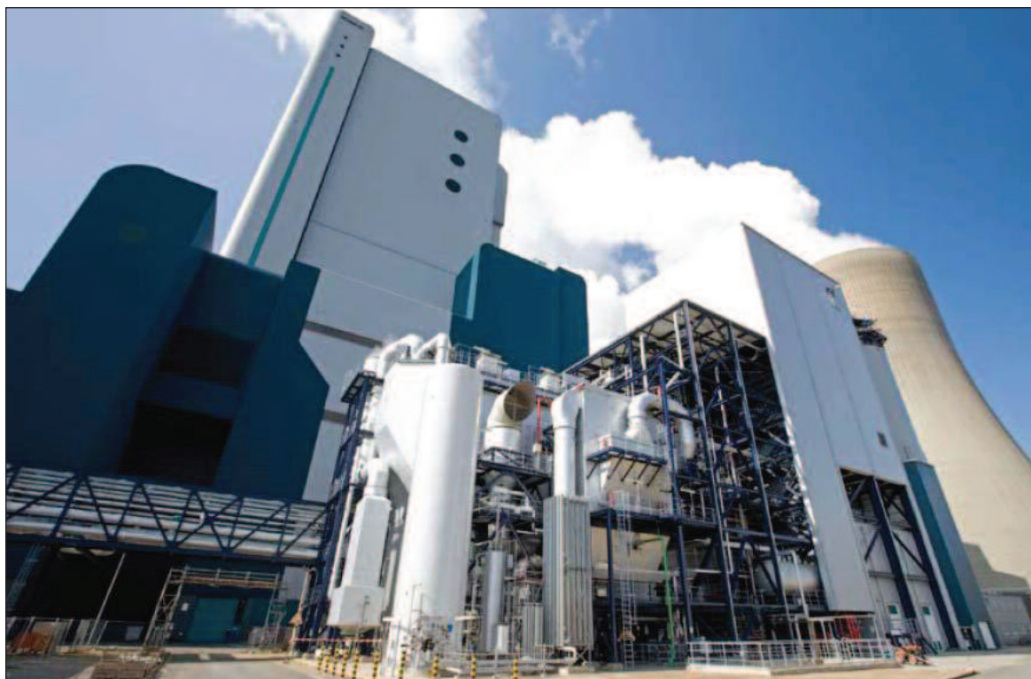
Figure 9 RWE's commercial prototype WTA dryer at the Niederaussem power plant in Germany (von Bargaen, 2012)
